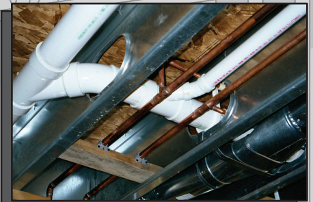
Wastewater, Supply and HVAC
