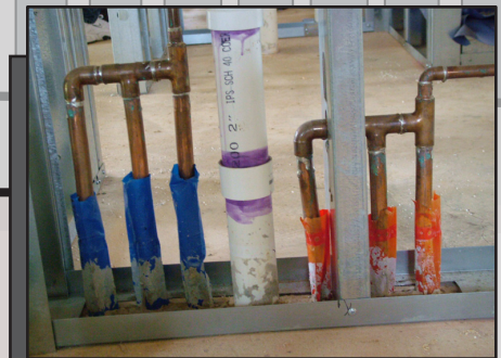
Cut Track with Copper and Wastewater
