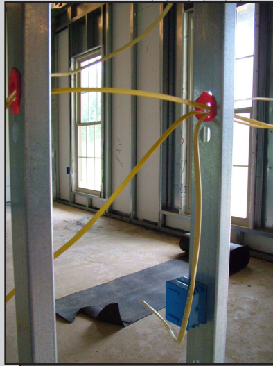
Electrical Box and Wiring
