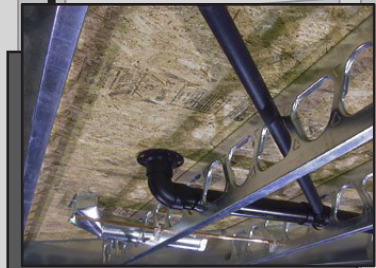
Wastewater and HVAC
