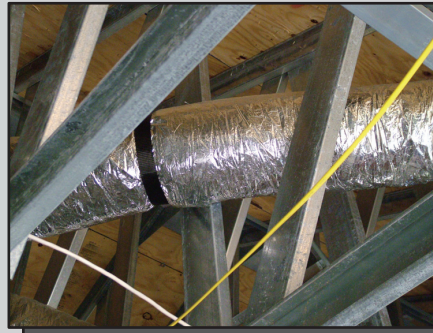
Insulated Duct in Attic
