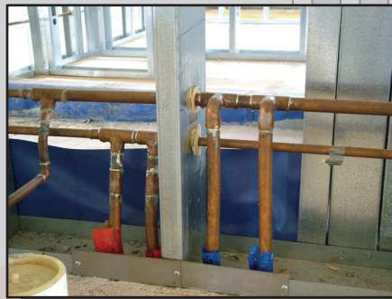
Copper Supply Pipes
